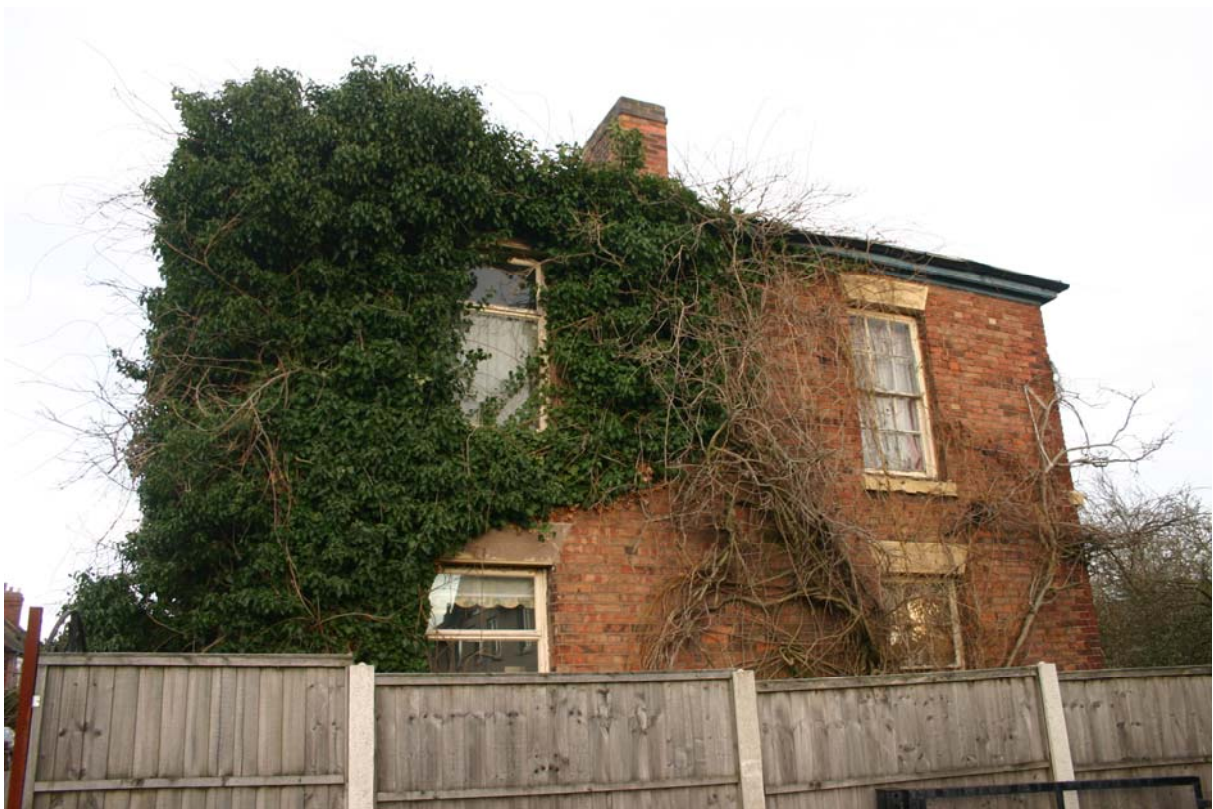
The locally listed Leys House, in poor condition externally
