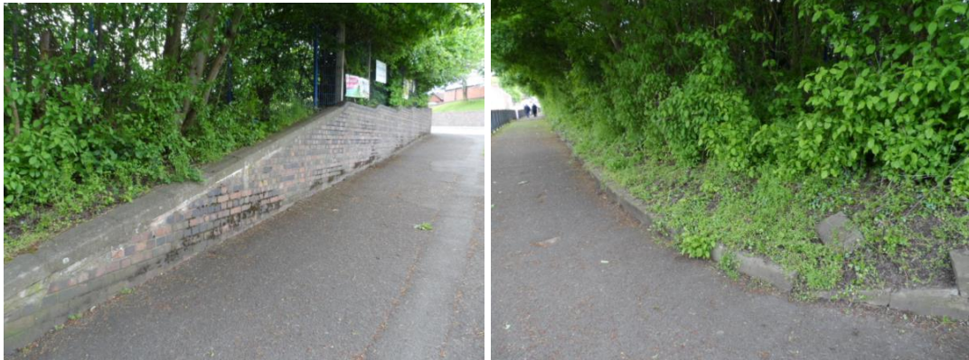
Figure 7 – Wall at the corner of Hockley and Watling Street requires cleaning and repairing of wall
